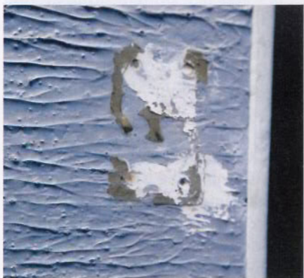
Leaks can occur via unused bolt holes that have been caulked over.
