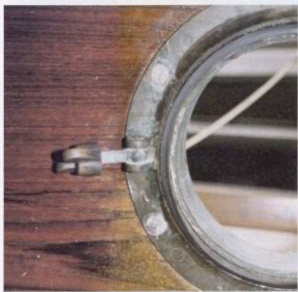
Water ingress has caused the veneer to lift and the wood to stain around this porthole.
