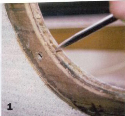
1 To repair a porthole leak, first remove the balsa core from around the portlight opening.
